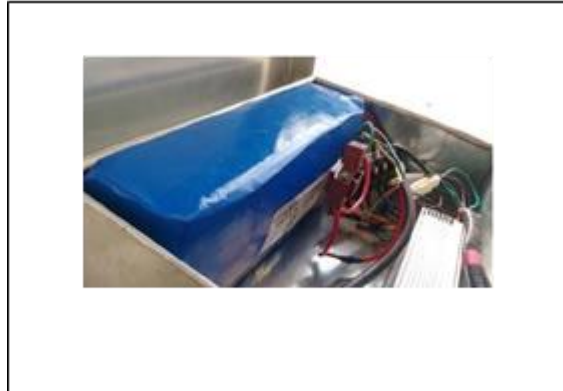
Fig. 6. Tractive Accumulator Mounting at Scooty Front Foot place
